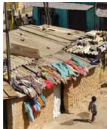
Typical asbestos cement roofing in a slum in India. Note the lack of indoor ventilation, apart from that available by the doorway. (Photo: Nick Clarke)
