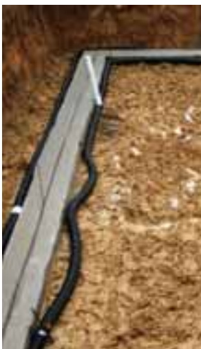
Venting the soil under and around a home helps prevent radon gas from seeping into floors. (Photo: Cincinnati Habitat for Humanity: http://cincinnatihabitat.org )
