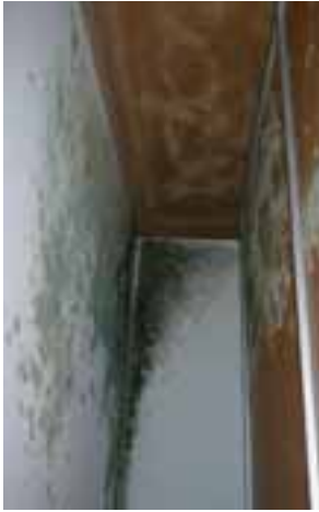
Mould on residential ceiling and wall. (Photo: Juergen Rath)
