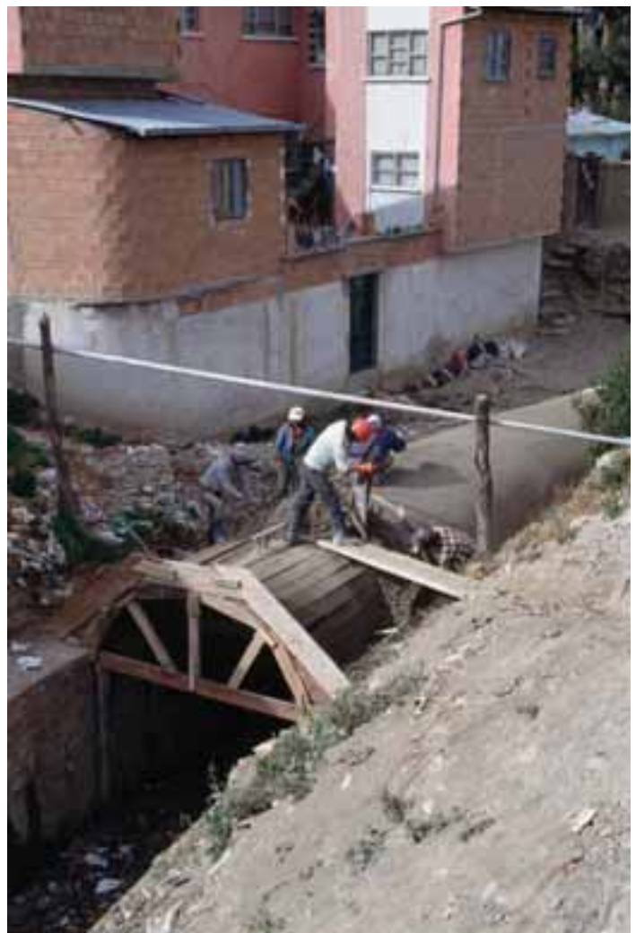
Building a closed sewage line over an open waste stream in a new neighborhood on the outskirts of Cochabamba City, Bolivia. (Photo: © Mark Edwards, Hard Rain Picture Library)
